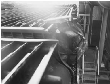
FIGURE 21.5 Poor control of aerosol release from a cooling tower.
