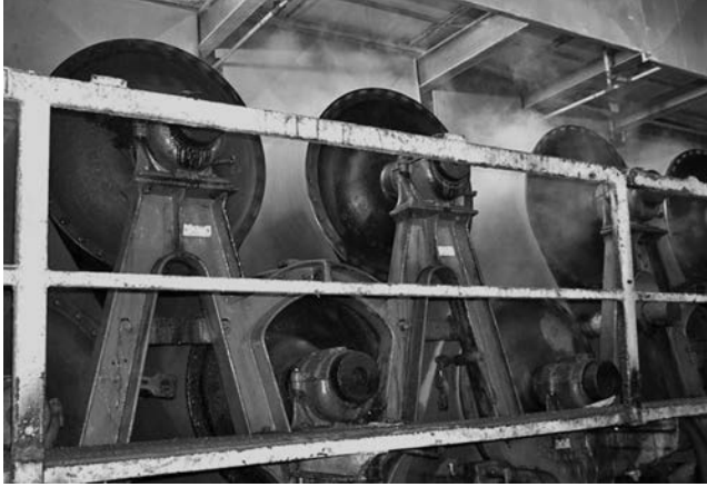
FIGURE 32.18 Steam heated dryers evaporating the remaining water.
