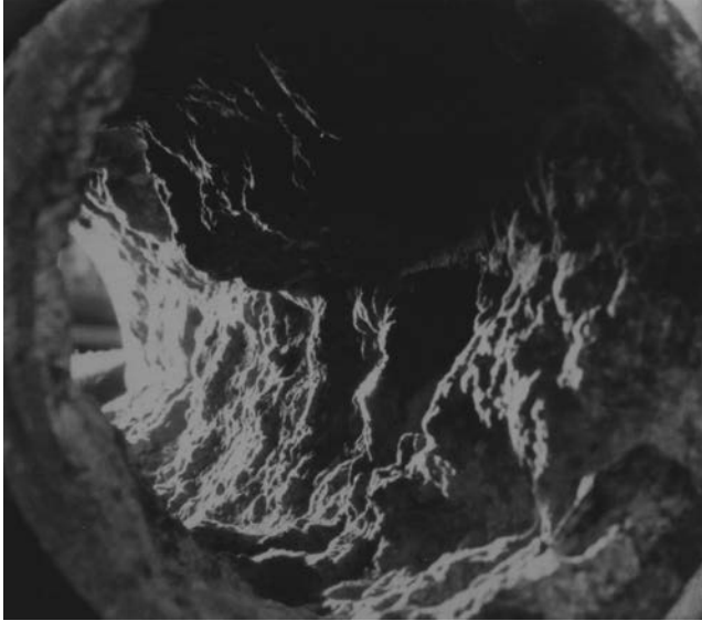
FIGURE 15.21 Corrosion products containing iron oxides on a steel pipe can create voluminous deposits, almost plugging this utility service water pipe.
