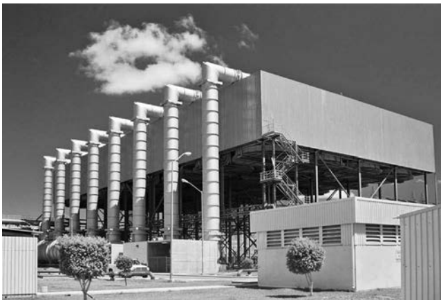
FIGURE 33.23 Typical dry cooling tower. (Courtesy of SPX Cooling Technologies, Inc.)
