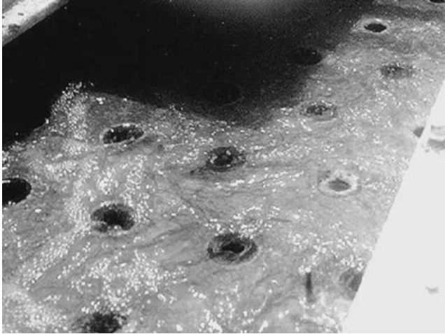
FIGURE 18.19 Open-deck cooling tower showing clean water distribution orifices and appropriate water level.
