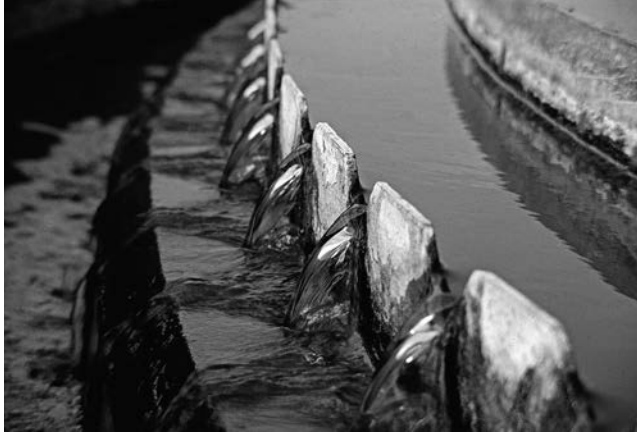
FIGURE 5.10 A clarifier can effectively remove the majority of suspended solids and humic matter from raw water as illustrated by the output water.
