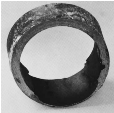
FIGURE 13.2 Carbon dioxide corrosion.
