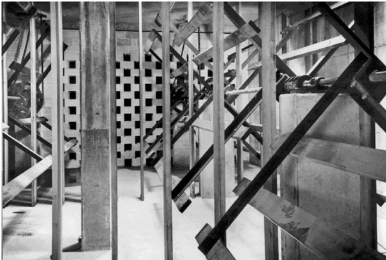
FIGURE 6.17 Reel-type paddle flocculator. (Courtesy of Envirex, a Rexnord Company.)
