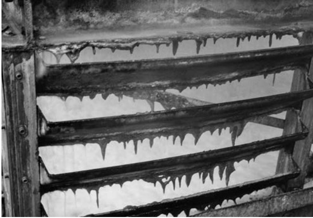
FIGURE 17.14 Example of biofilm hanging on water-wetted louvers near the basin of a cooling tower. The biofilm may contain bacteria, fungi, and inorganic material. If the biofilm falls off the louvers, plugging of heat exchanger tubes can occur.
