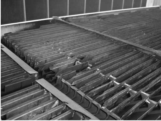
FIGURE 21.4 Damaged drift eliminators are a potential problem for aerosol release.
