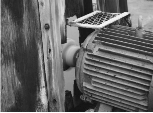
FIGURE 30.10 Air leakage can occur through holes and gaps in the fan stack.
