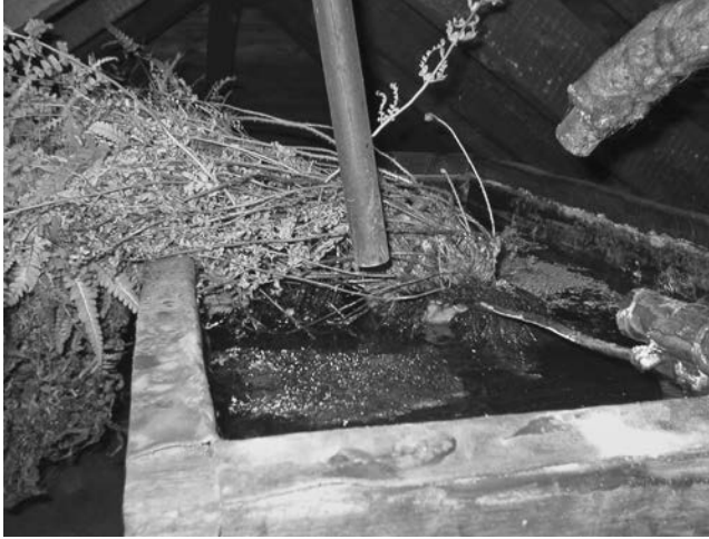
FIGURE 21.7 Poorly controlled system with excessive micro and macro biological growth.
