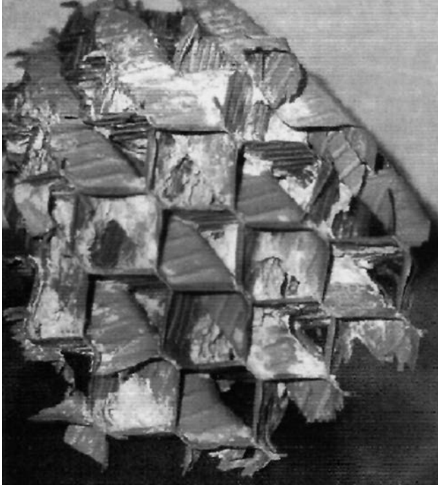
FIGURE 14.30 Heavy fouling of film fill caused by inorganic scale formation.
