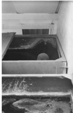
FIGURE 21.8 Contaminated section of system.
