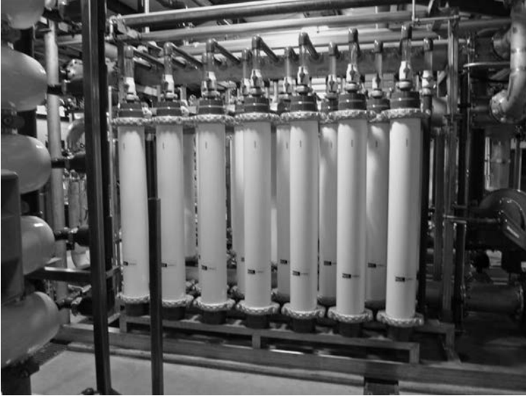
FIGURE 8.21 Ultrafiltration skid showing clear permeate piping.
