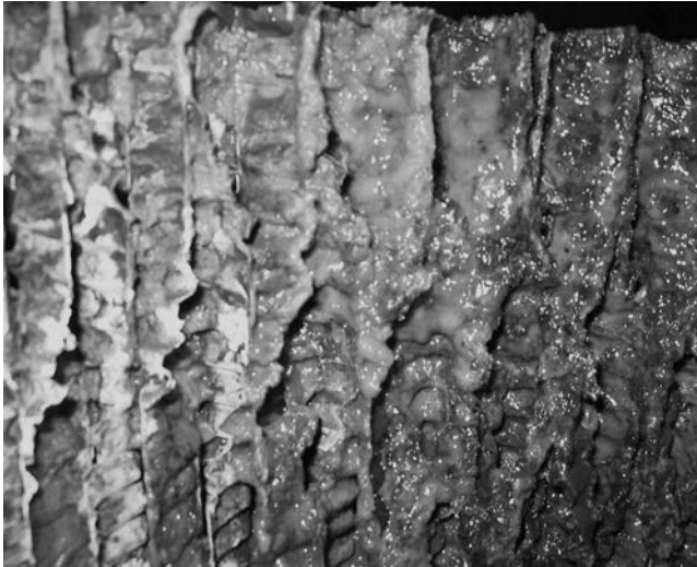
FIGURE 21.2 Biofilm in tower fill.
