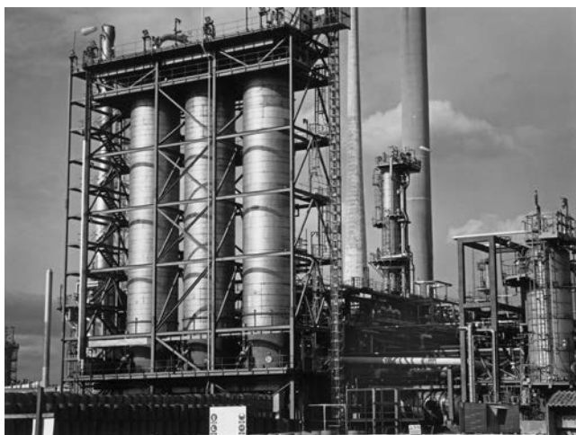
FIGURE 35.17 Vacuum residue hydrotreater reactors.
