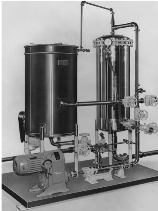
FIGURE 40.4 Typical filter installation in the food and beverage industry. Note the use of special stainless steel piping and fittings. (Courtesy of Croll-Reynolds Engineering Company, Inc.)
