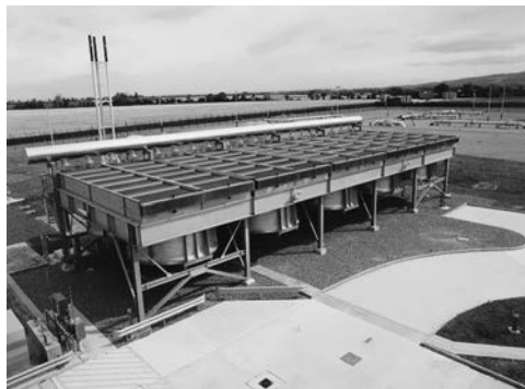
FIGURE 14.25 A fin-fan cooler with two circular fans mounted under the bank of tubes that carries the hot process fluid. (Courtesy of SPX Cooling Technologies, Inc.)
