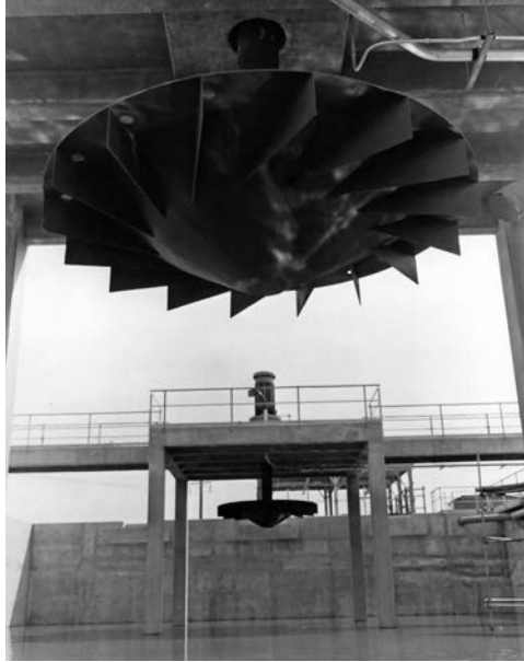
FIGURE 29.10 Details of construction of a fixed-position surface aerator, shaped to produce high-volume pumping and air entrainment. (Courtesy of Infilco Degremont Inc.)
