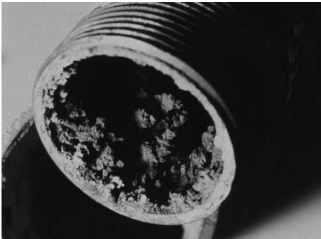
FIGURE 17.6 Iron-depositing bacteria within tubercles contributed to the voluminous iron oxide deposition in this steel distribution pipe.
