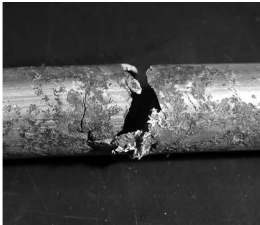
FIGURE 16.24 Example of severe stress corrosion cracking on a stainless steel pipe.
