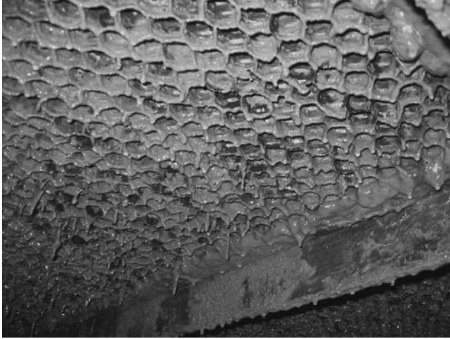
FIGURE 21.3 Severe biofilm on the underside of tower fill.
