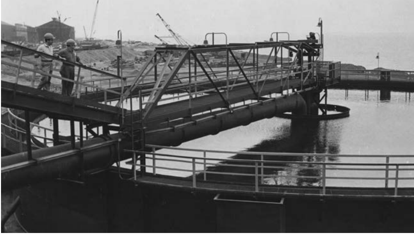
FIGURE 38.3 Clarifier-thickener used to treat blast furnace gas scrubber water and to recover solids. (Courtesy of Inland Steel Company.)
