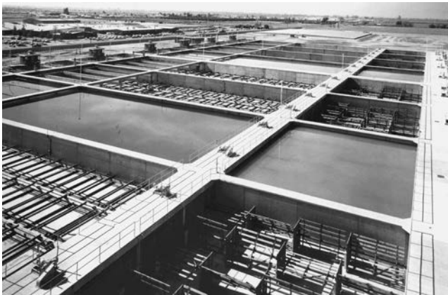
FIGURE 6.19 Conventional water treatment plant showing reel-type flocculation units, rectangular sedimentation basins in parallel with common wall construction, and sludge collection flights. Final filtration is not shown. (Courtesy of FMC Corporation.)
