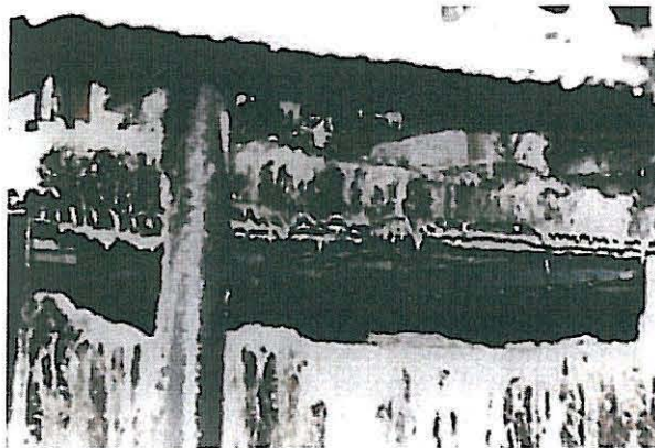
Figure 4-8. Microbiological slime in a cooling tower.
