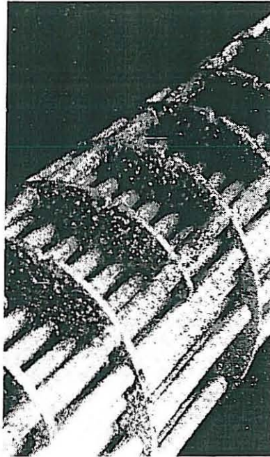
Figure 4-10. General corrosion of tube bundle baffles.
